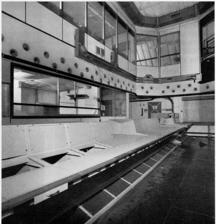
Two-level control room. Photo: Nick Catford
